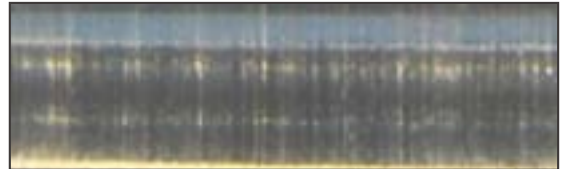
深さ100mm付近の状態 Condition at depth of around 100mm
